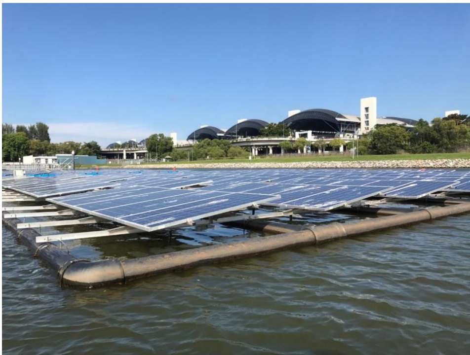
Floating solar panels at Tengeh Reservoir
